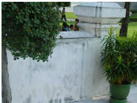
Figure 11 Moisture and Crack
