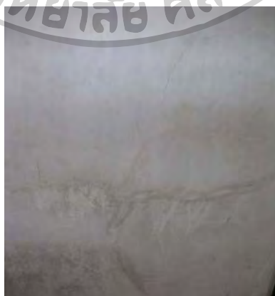
Figure 10 Minor Crack inside the Throne Hall
