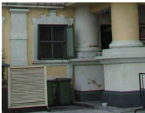
Figure 16. Small cracks and moistures at the base of the column / Building A.
